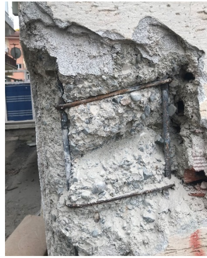
d) Yetersiz dozajlı beton
